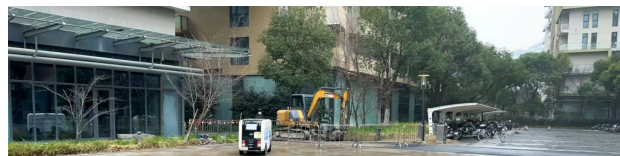
Notice about Emergency Repair of Sewage Pipes on the East Side of the Silk Road Canteen and Road Closures
